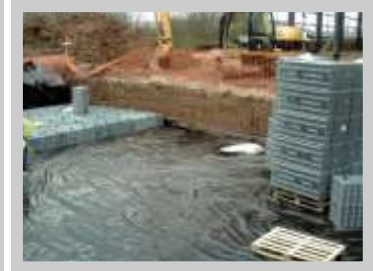
SUDS Drainage Attenuation System
