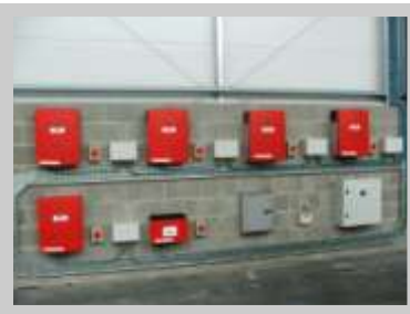
Photo Voltaic Invertors, Meters & Controls
