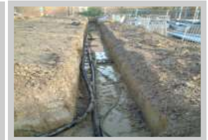
Ground Source Heat Pump Bore Field
