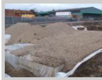
SUDS Water Attenuation
